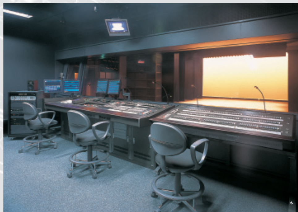
▼中劇場調光室 THEATRE lighting control room
